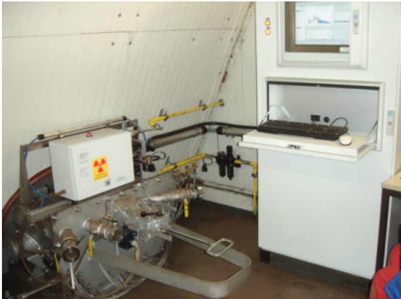
Measuring system converter dust
